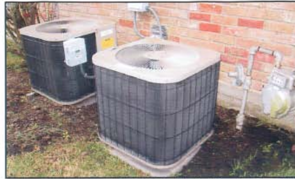
Exterior Residential Condensing Unit
